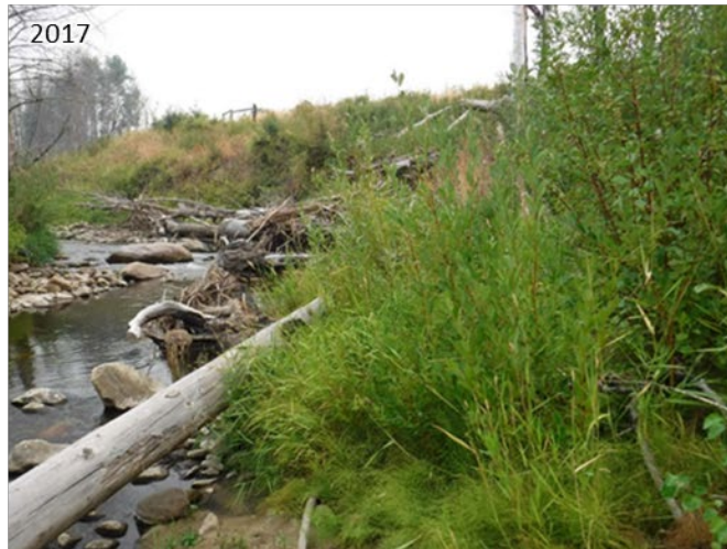
Figure 3-35. Site D looking upstream. Upper left: immediately post-construction (2013). Upper right: post-fire, post-5-year flow event (2014). Bottom: post-7.5-year flow event (2017).
