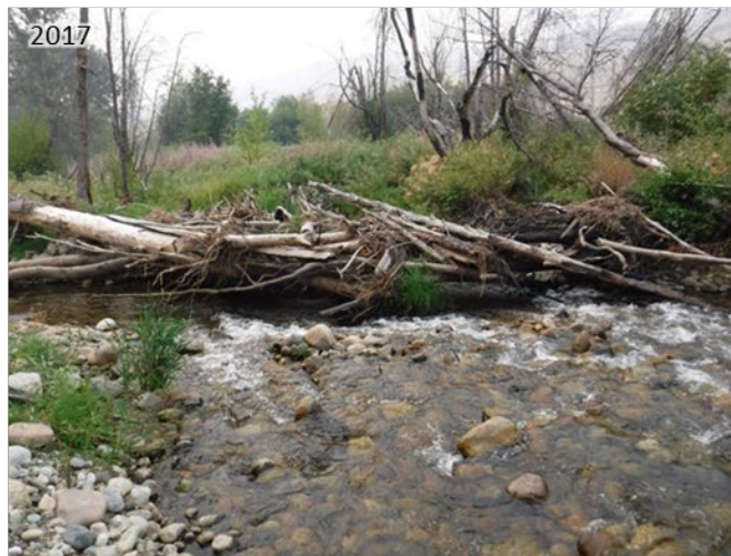
Figure 3-42. Site K Looking at the face of the structure. Upper left: immediately post-construction (2013). Upper right: post-fire, post-5-year flow event (2014). Bottom: post-7.5-year flow event (2017).
